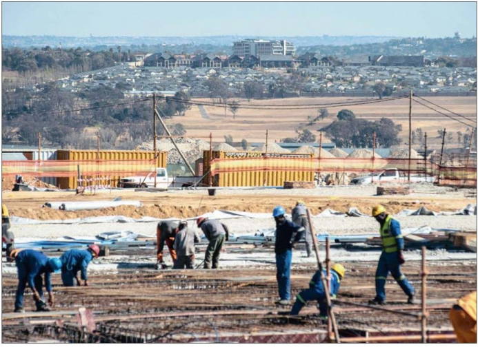
Workers arrange steel reinforcement rods during the construction of the Mall of Africa retail space at the Waterfall City residential and commercial urban development. PHOTO: BLOOMBERG
